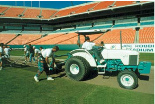
West Coast Turf installs thick-cut, big-rolls of Tifway II for Super Bowl XXIX, Joe Robbie Stadium, Miami, FL.
