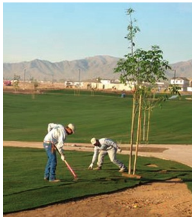
Workers put finishing touches on a recent West Coast Turf sod installation at Marley Park.
